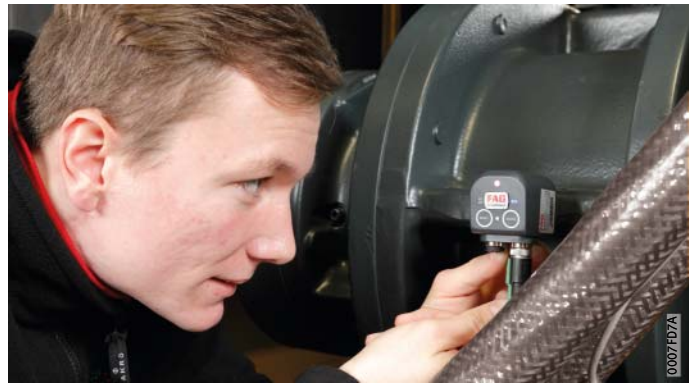
Figure 3 Commissioning of FAG SmartCheck
